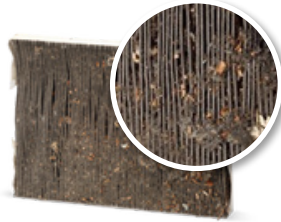
Without A /C maintenance
